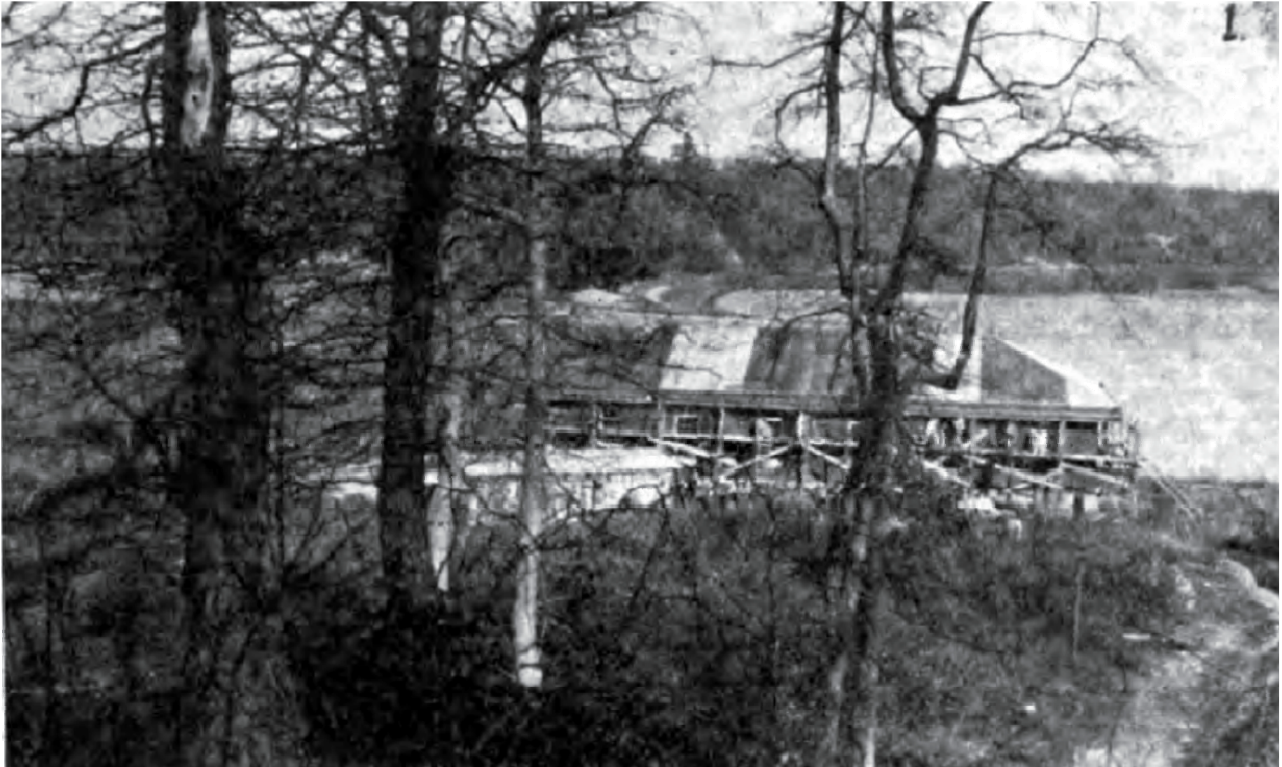
The operations building under construction. The construction shack in front of it is believed to be the locations of Edwin Armstrong's demonstration of his regenerative receiver to Marconi personnel on 30-31 January 1914.
